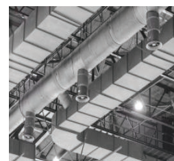
HVAC duct system
