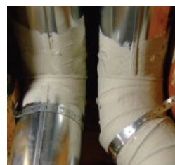
HVAC duct system
